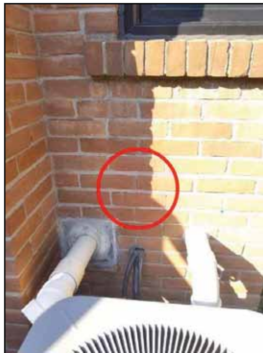
14. Missing electrical shutoff
