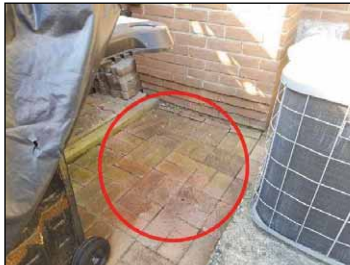
9. Low spot(s) in grading. Should be addressed...
