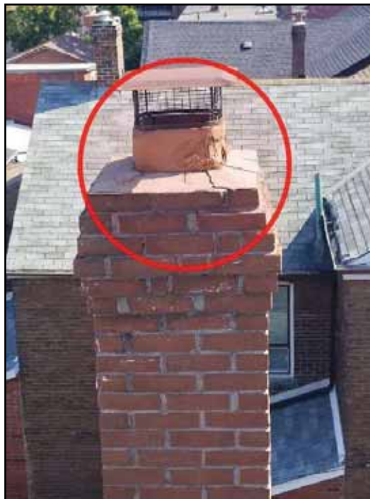
12. Damaged, cracked or deteriorated flue or...
