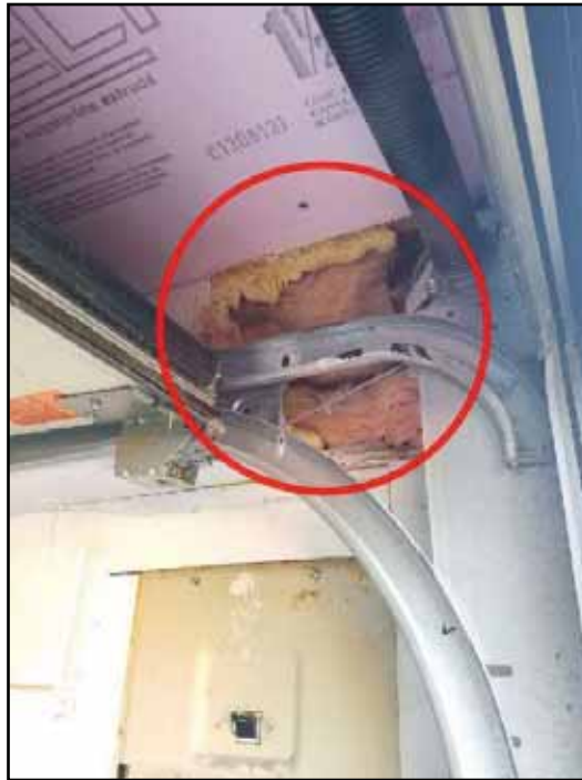
23. Gaps or cutouts in walls or ceilings need t...
