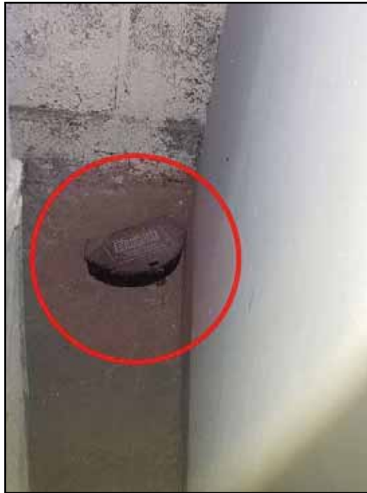
21. Evidence of previous pest/ rodent issues,...
