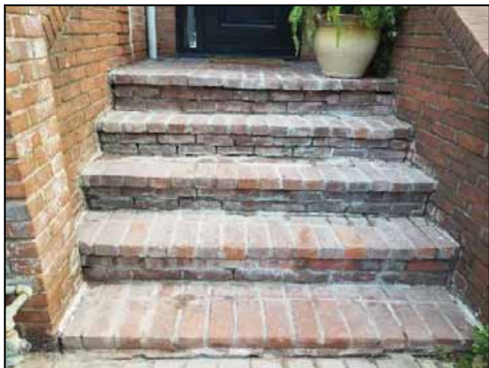
6. Masonry or concrete spalling
