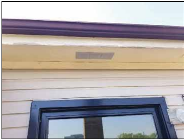
3. Paint - deteriorated / missing
